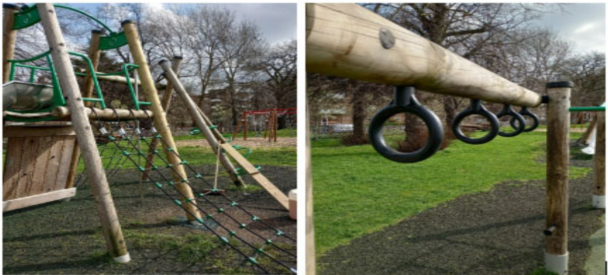
Figure 21: Hurlingham Park - Repairs to multi-play unit, eradicating issues from annual inspection reports. New ropes, and posts.
